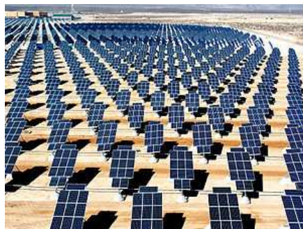
Nellis Solar Power Plant, the second largest photovoltaic power plant in North America
